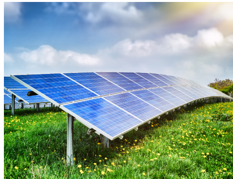
Solar Panel System
