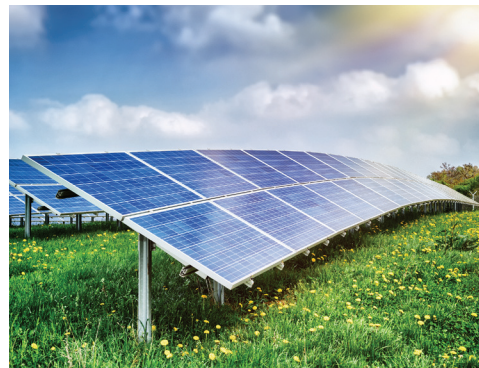
Solar Panel System
